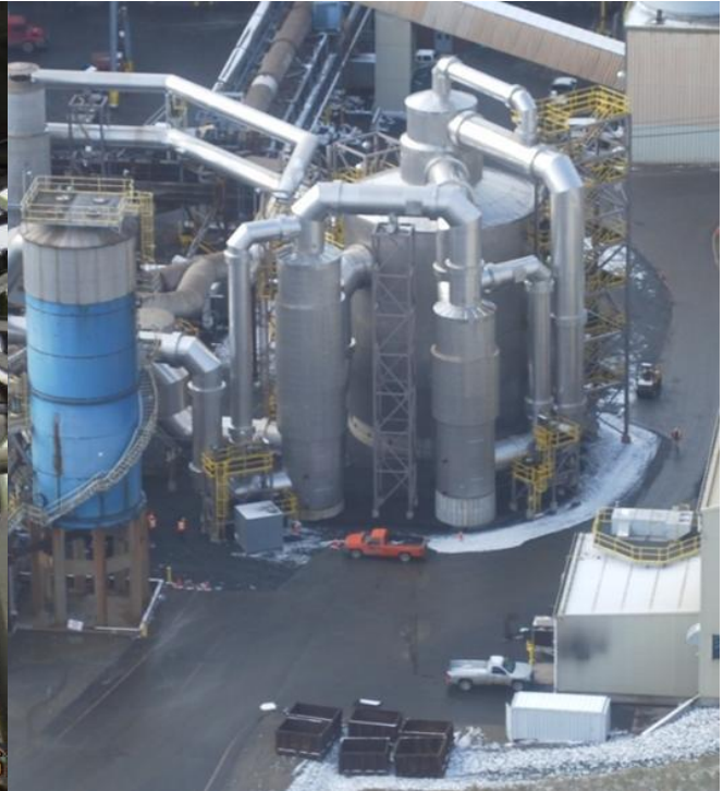
Figure 4. - New 4-pass converter in the acid plant to increase sulphur capture. (2012)
