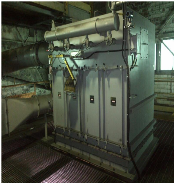
Figure 17. - New Dust Collector on the conveyor (2015)
