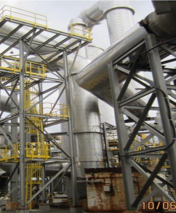
Figure 3. - New Tail Gas re-heater (2014)
