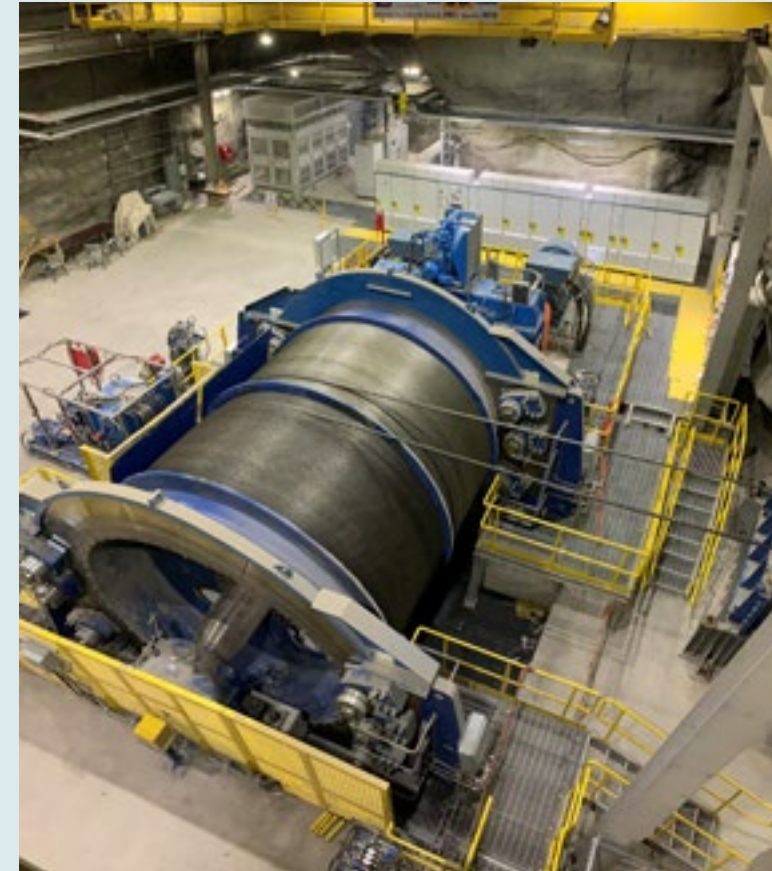
Headworks construction (complete) at the 1,150 m level underground. Photo above shows hoist commissioning: 300 Service Roped-up, and photo below shows hoist commissioning: 100 Production Hoist Roped-up.
